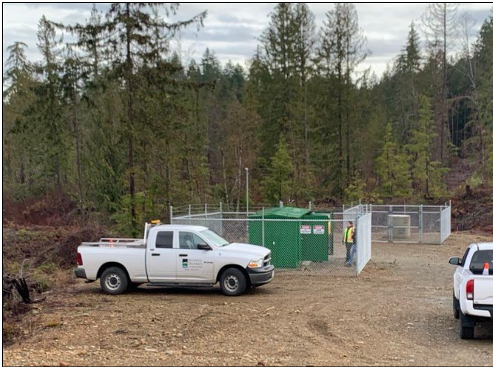
Whiskey Creek Well Site and UV Treatment kiosk
