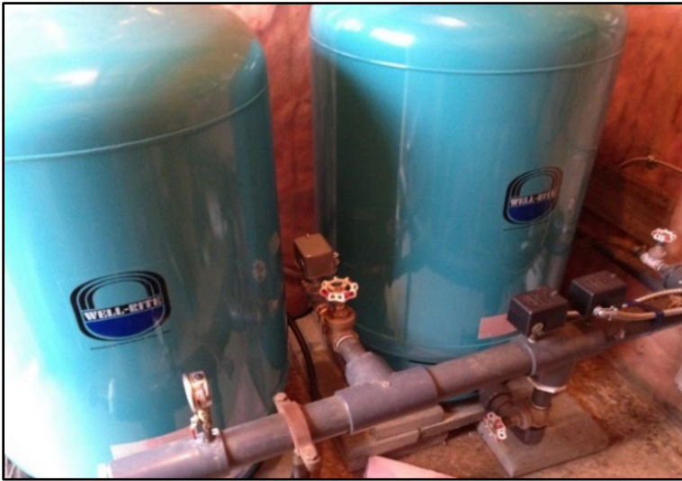
Pressure tanks inside the Westerne Heights pump house
