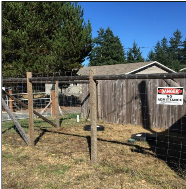
Westurne Heights Well Site and underground storage cisterns
