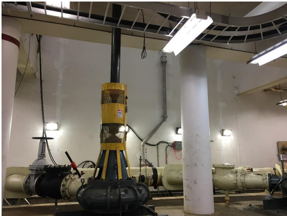
Figure 4-2 Piping Not Restrained
