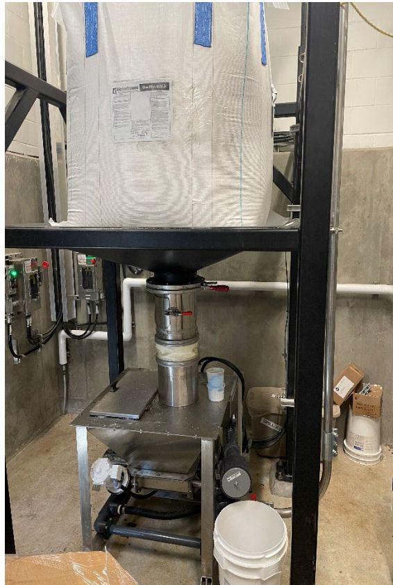
Figure 3– Dewatering Polymer Mixing and Chemical Delivery System
