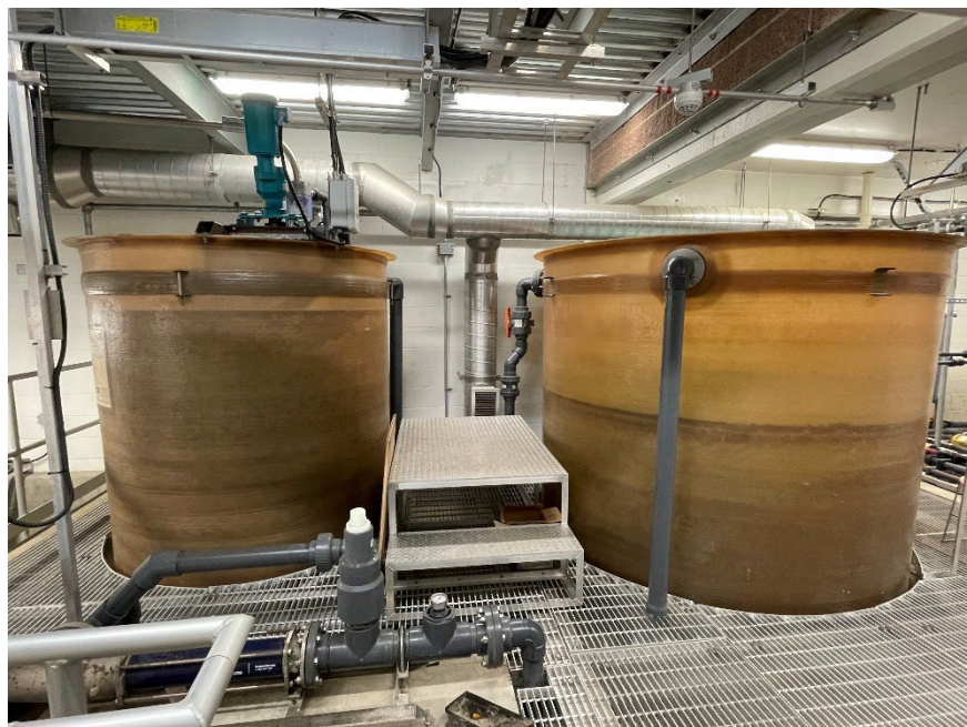
Figure 4– Dewatering Polymer Mixing and Chemical Delivery System
