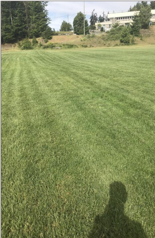
Photo 6: Depression in Field
