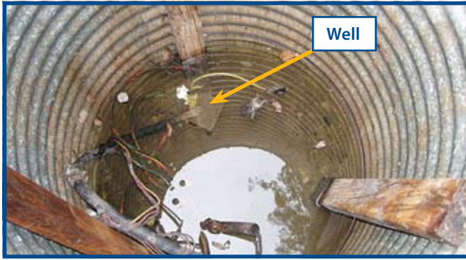
Figure 3. Water and debris in well pit
