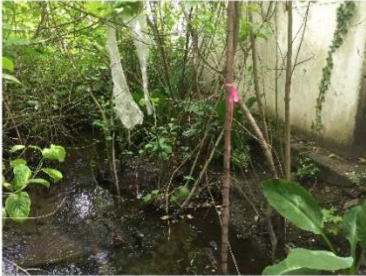
1.) R2 - ditch line along side of 7-11 is poor.
