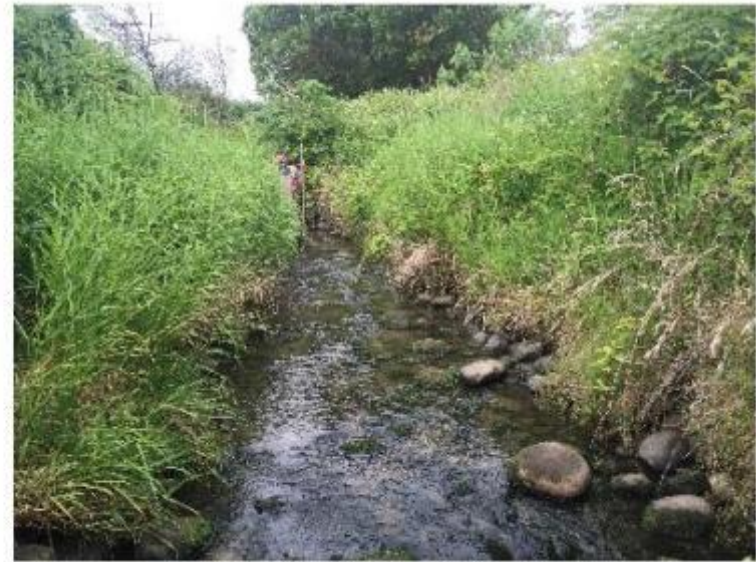
3.) R1 above culvert needs trees and gravel
