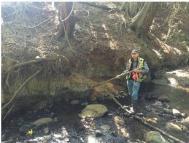
2.) Bank erosion below Newton st.
