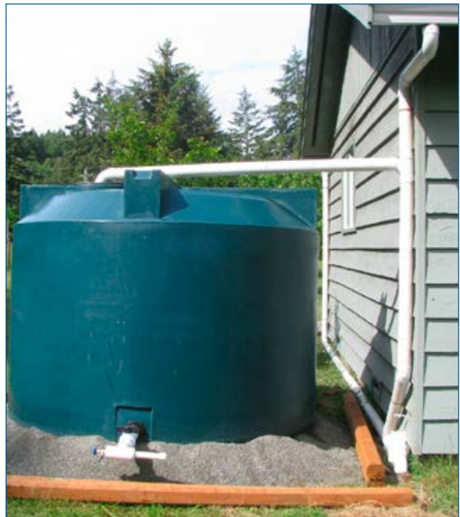
Two 7,550L tanks with interconnecting piping and protective valve boxes (before final backfill).
