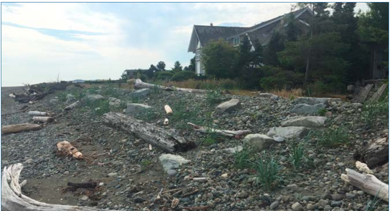
Completed Green Shores project in Parksville, BC, to regrade and stabilize eroding shore line
