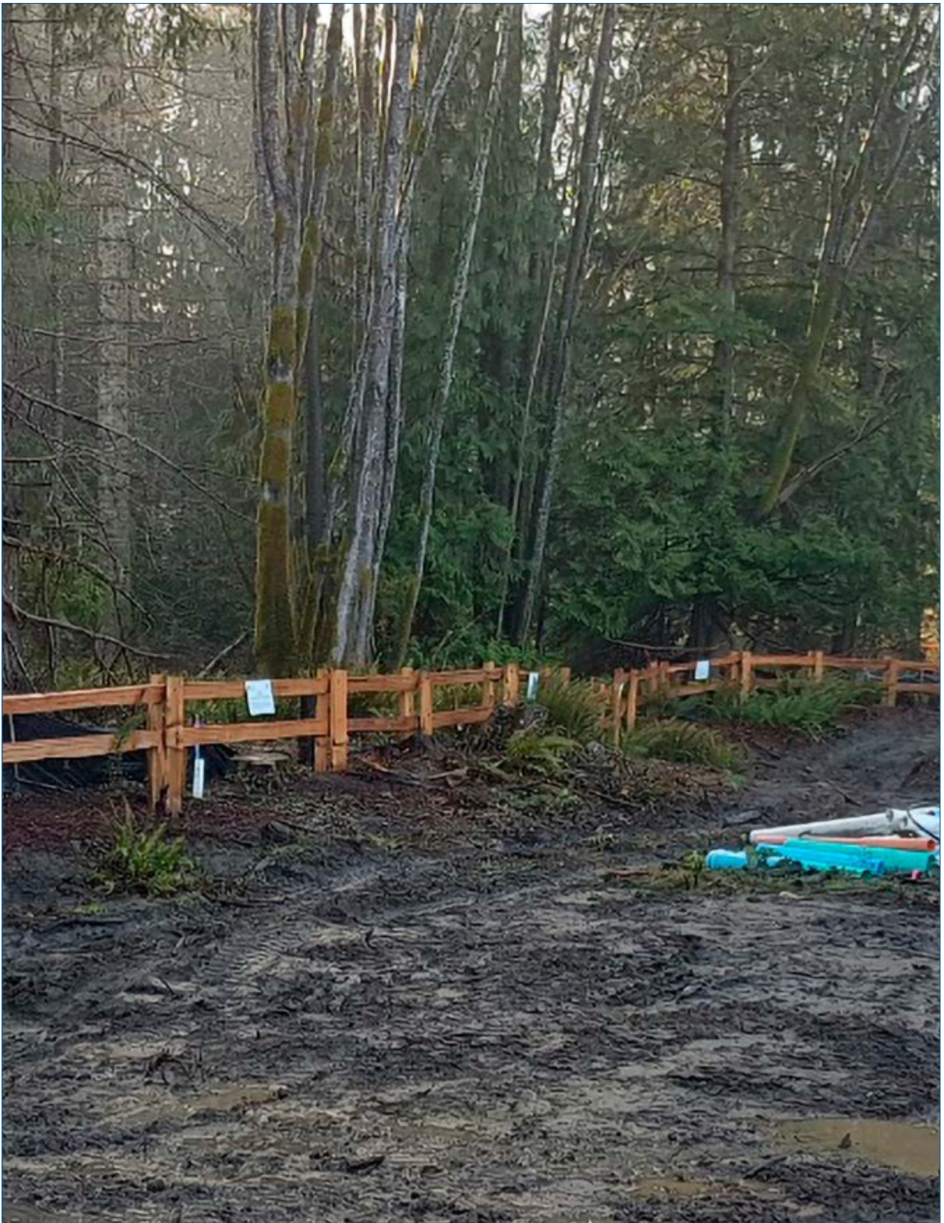
Permanent fencing to protect the riparian area of French Creek in place before residential construction began
