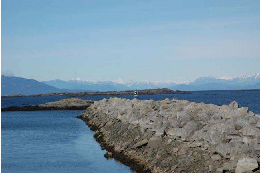
Figure 14: View of the protected southwest side of the breakwater, looking north from Schooner House. Note slightly finer fill material on the lower slope of the breakwater.
