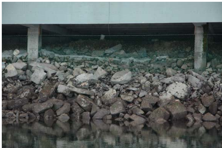
Figure 8: Rubble and fill under hotel pilings.
