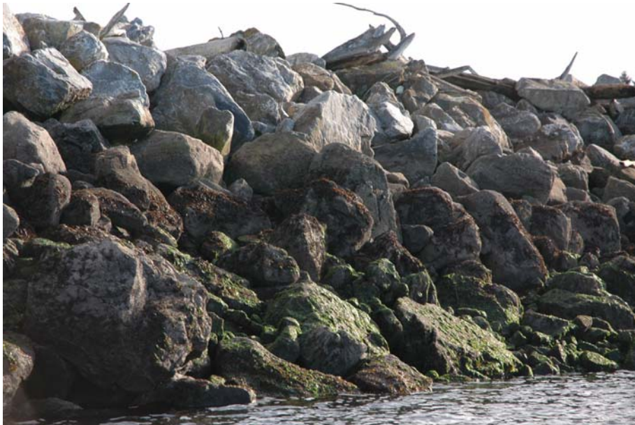
Figure 15: East facing, high-energy side of the breakwater, showing coarse riprap and log debris on the top of the berm.
